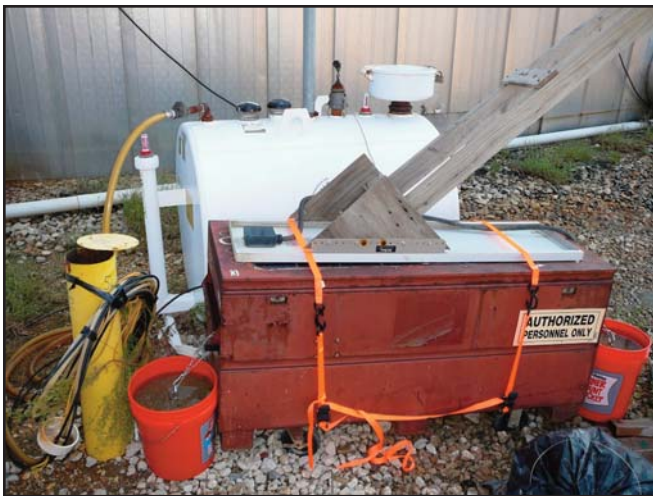
Well, tank, well equipment box & solar panel strapped down
